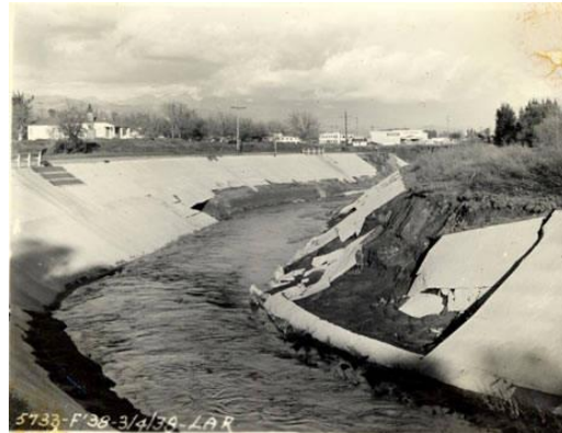
Levee failures along the Los Angeles River
